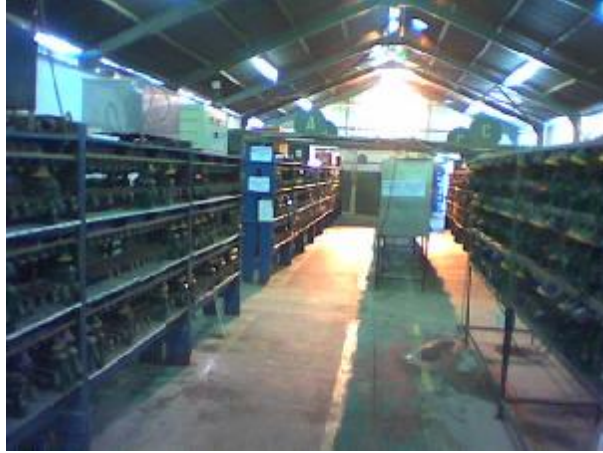
Typical Lamp room with battery charger racks
